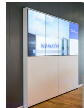
Slim Video wall with 4 x 55" displays, perfectly integrated into the highly representative lobby.
